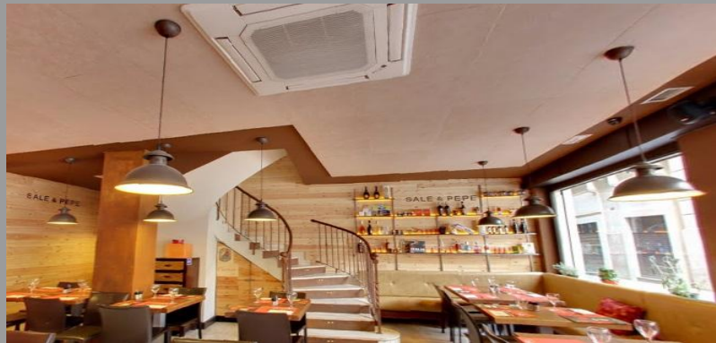
Acoustic Panels on ceiling.
